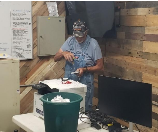
Eddie – Wiring shop office
