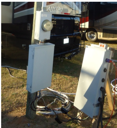
Meter base mounted on pole with 200 amp power breaker panel underneath meter for which your ministry is responsible. On the right is ALCOM provided distribution panel. We also provide the cable between your breaker panel and our distribution panel.
