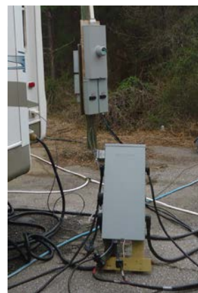
Another situation – note this site has 2-200 amp power breaker panels underneath one meter. Sitting in foreground is the ALCOM provided distribution panel with a second ALCOM panel out of site to the left. We can supply cable to extend approx 50' from meter to our panel. ALCOM normally connects our panel to your breaker panel.
