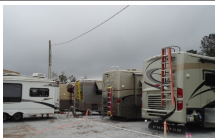
Some of our rigs are 13' tall. Please ensure your power poles and supply cables are sufficiently high for RV's to safely pass underneath.
